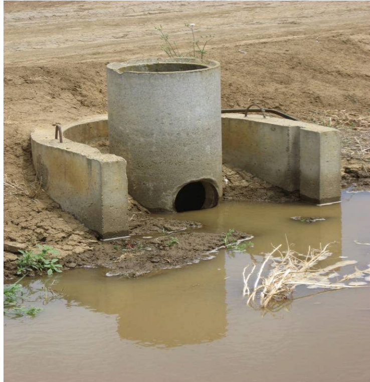
Figure 8. Field Drain at end of Sediment Basin
